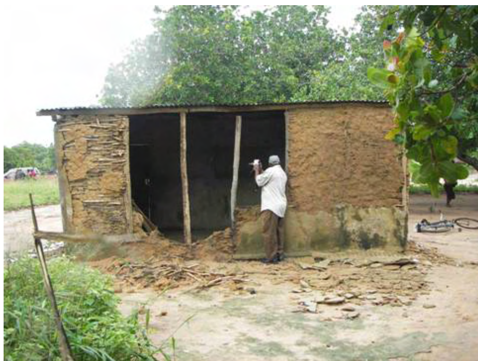
Figure 7 Partial collapse of a badly deteriorated wattle-and-daub dwelling. Most houses constructed from this material performed very well in the earthquake.
