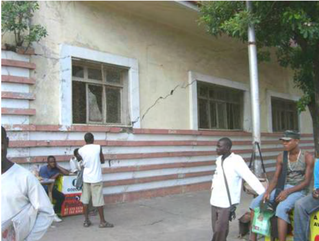
Figure 8 Major shear crack in a building in Beira, more than 200 km from the epicentre.
